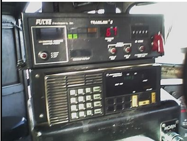
The typical “Wilma”, head-of-train (HOT) device (HTD), displays the current brake line pressure on the rear end.
