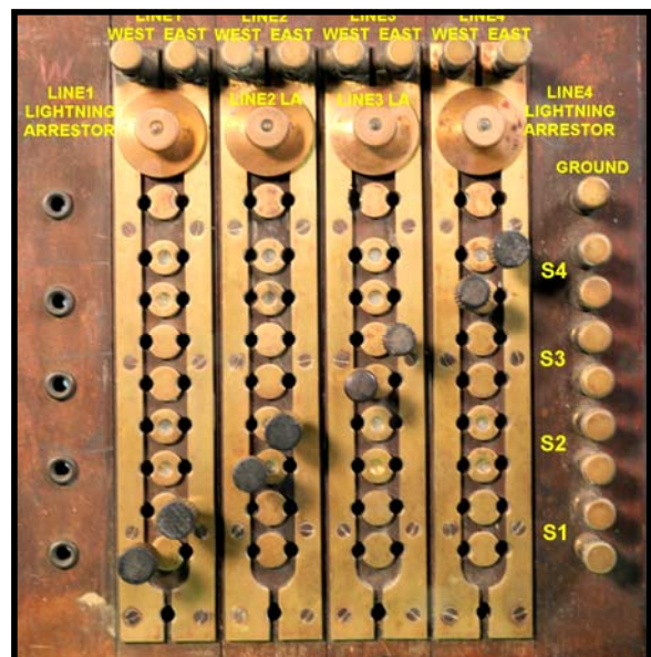
Figure 7. Four Line Telegraph Switch Board
